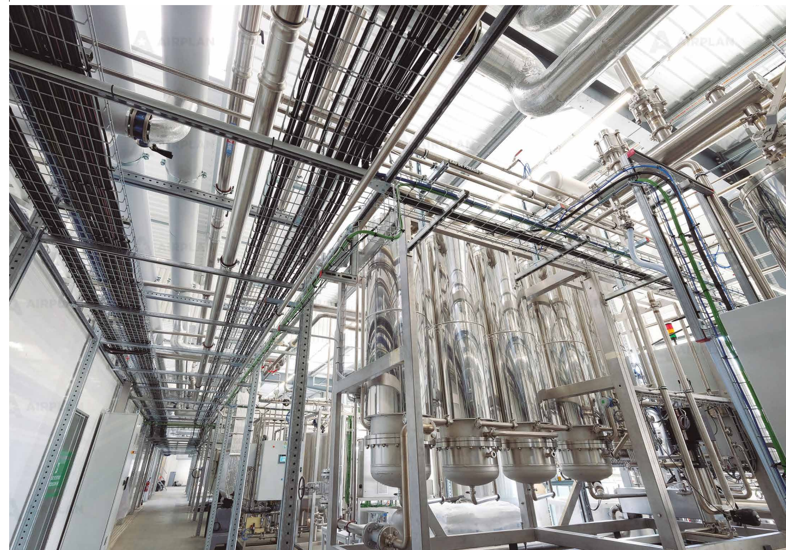
Clean Media / Black Utilities
